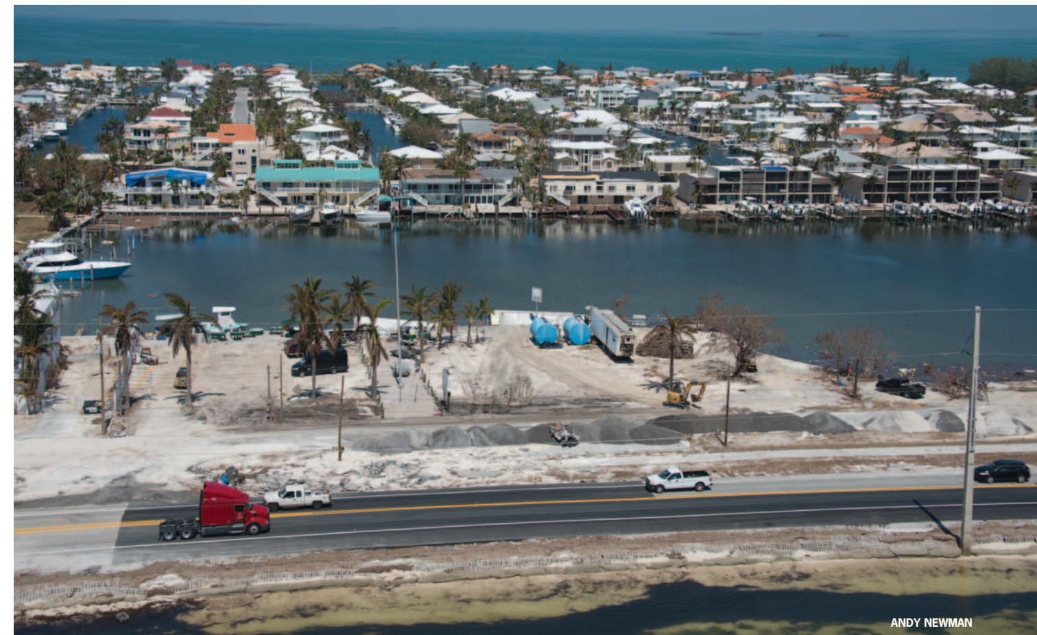
The Florida Department of Transportation restored about 150 feet of the Overseas Highway in Islamorada just four days after Irma eroded portions of the road.
